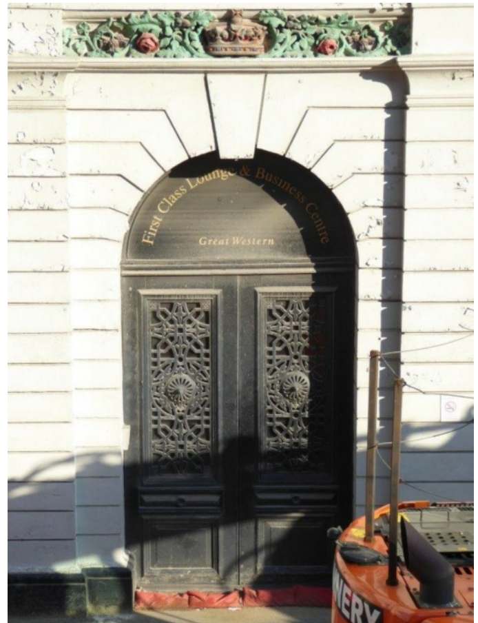
The 'royal door' used by Queen Victoria leaving the Royal lounge onto the original station platform
